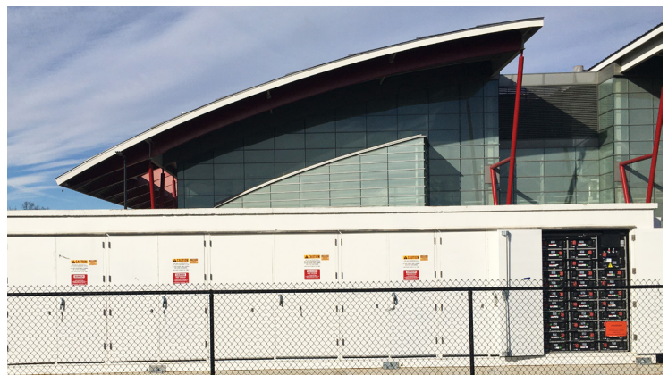
Battery storage on-site at UMASS Amherst
